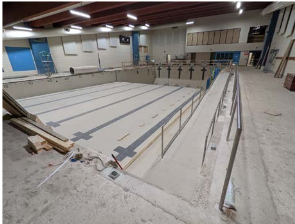
Interior: Work is in progress for the new submerged accessible ramp within Kinsmen Pool
