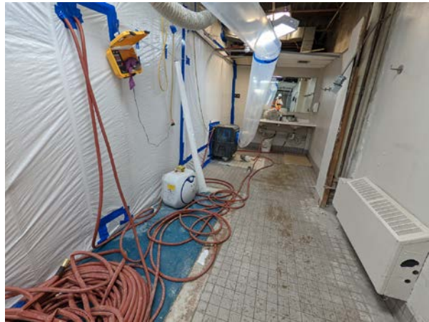
Interior: Demolition work within the Health Club washroom area is underway to expand the workout area
